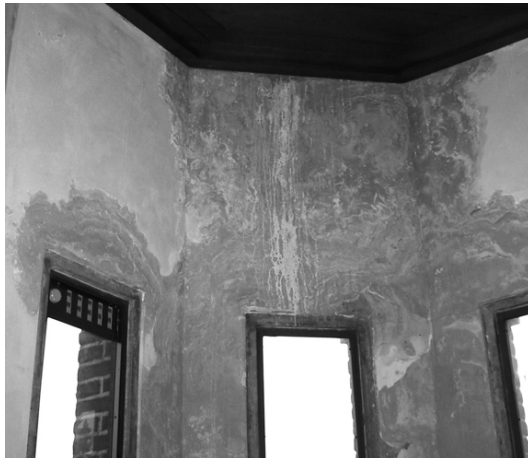
Figure 2. Moisture damage at the inside of the tower
