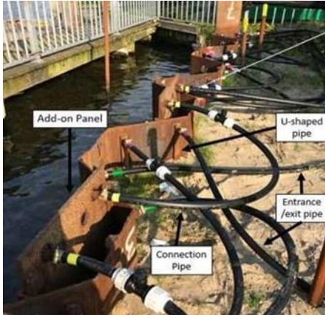
Figure 1. EQW case study installed in Delft (NL)
