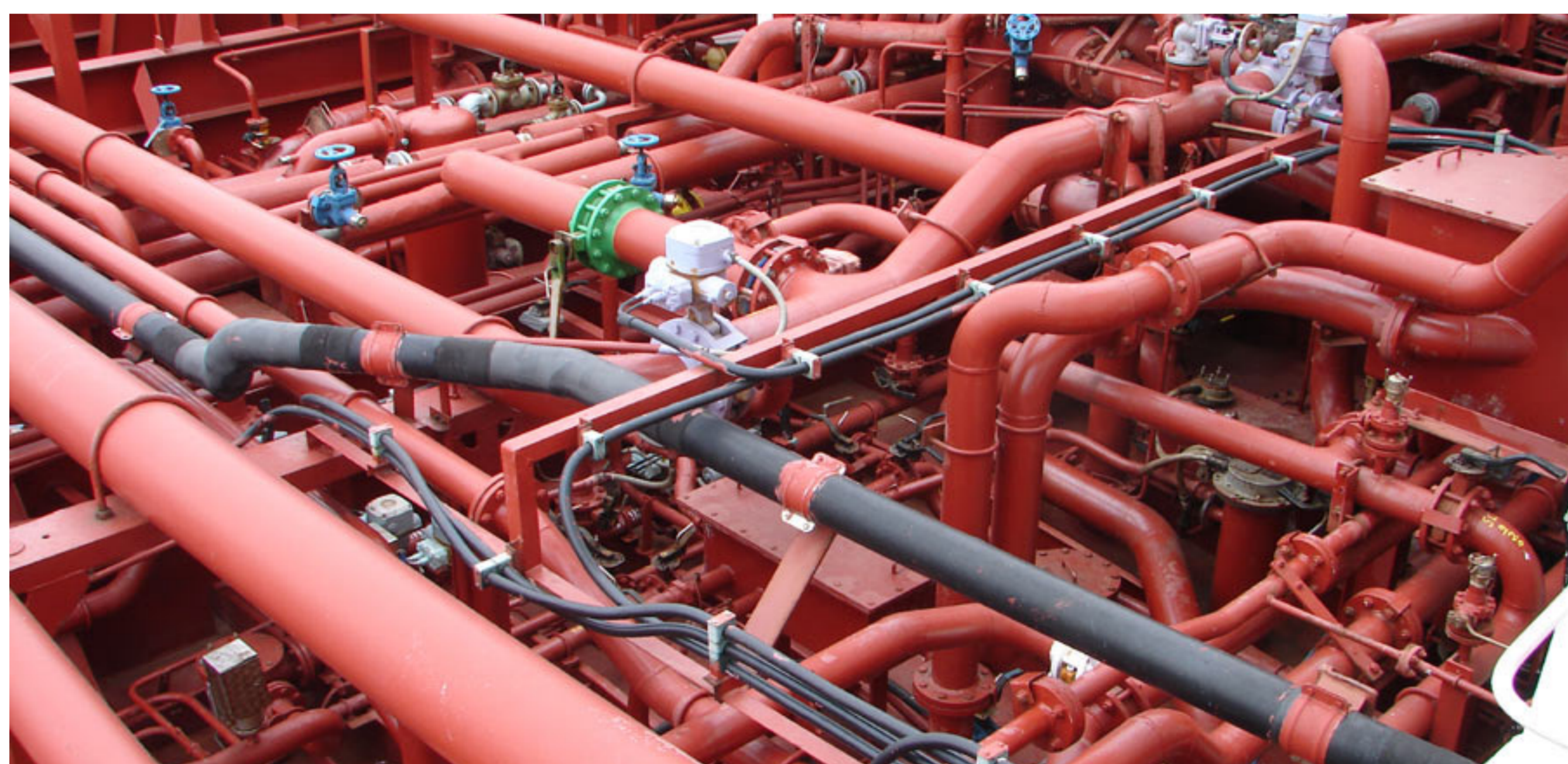
FIGURE 1. Piping systems on an oil/chemical tanker. Image licensed under CC BY-SA 3.0 via Wikimedia Commons.
