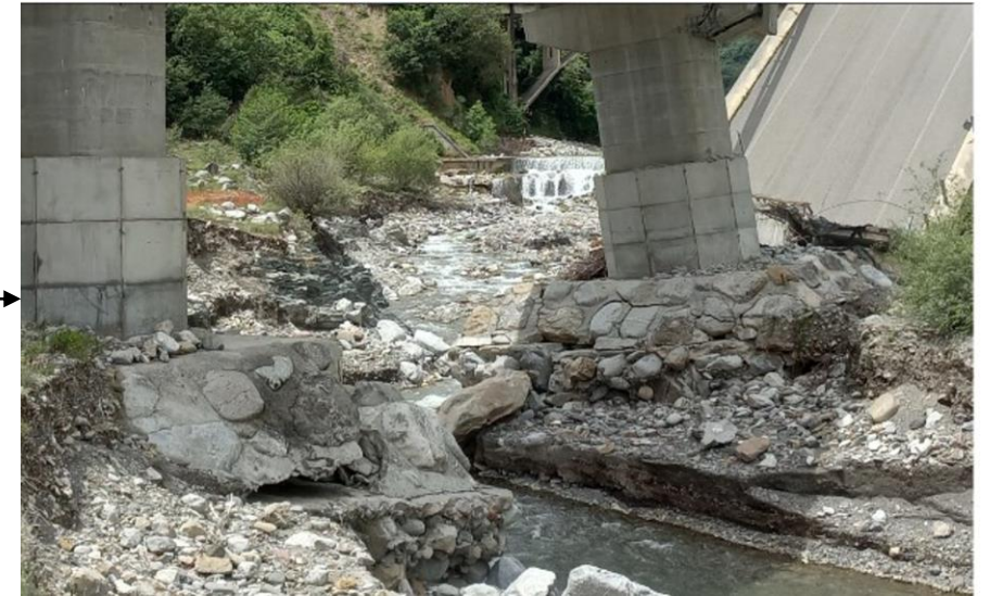
Collapse of the Longobucco bridge, (Cosenza, 2023)
