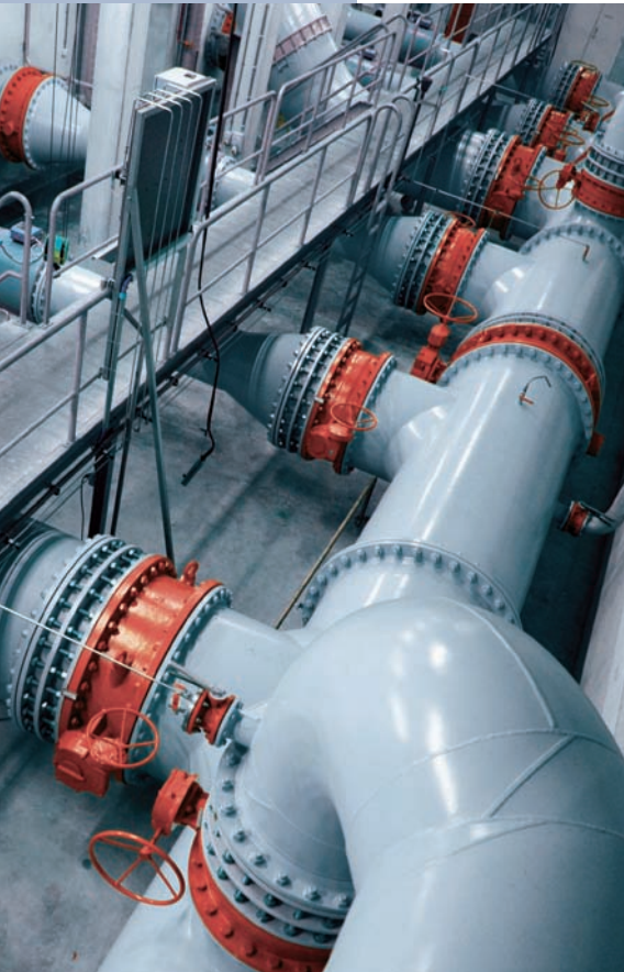
FIGURE 3: In the header assembly for the turbulent ozone reactors, filtered water passes through large pipes and empties into a long conduit or header roughly 1 m in diameter. The header mixes the filtered water and feeds it into the turbulent ozone reactors through relatively small pipes or “streets.”
